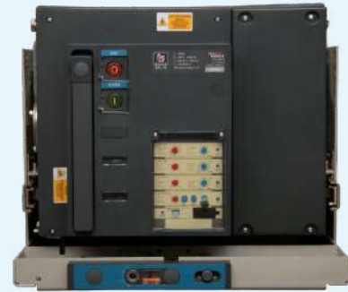
Mega power S1 ACB
